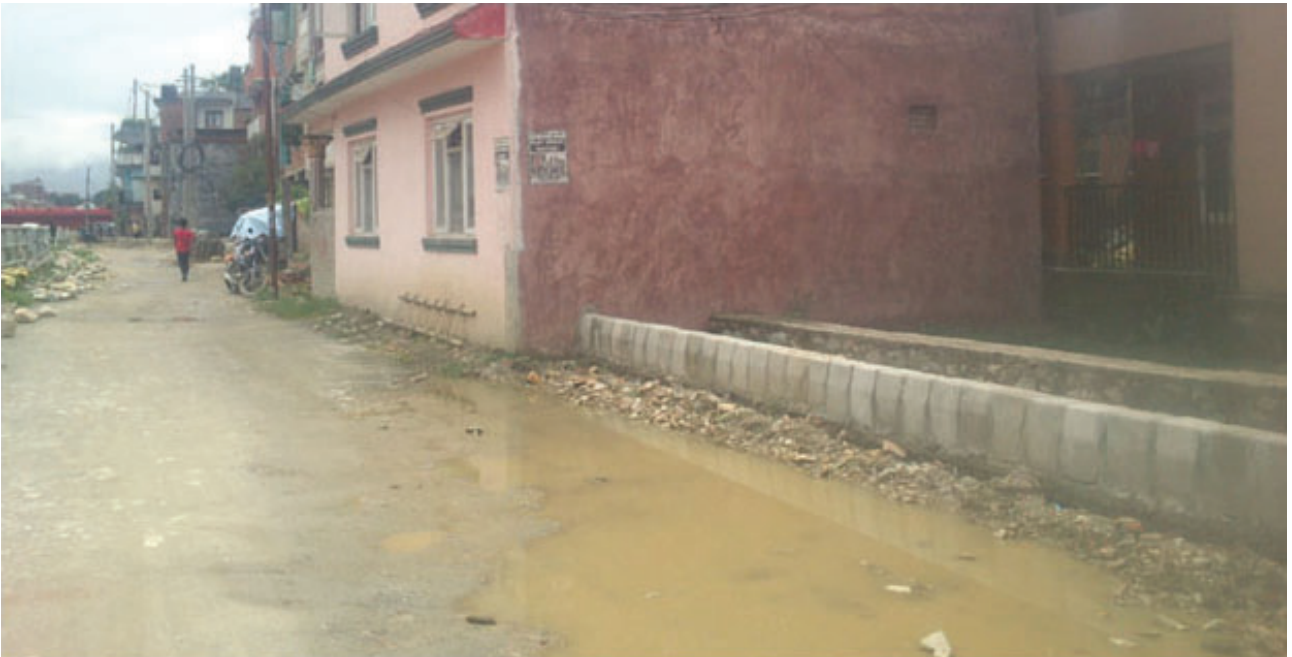
Figure 23: Encroachment by residential buildings
