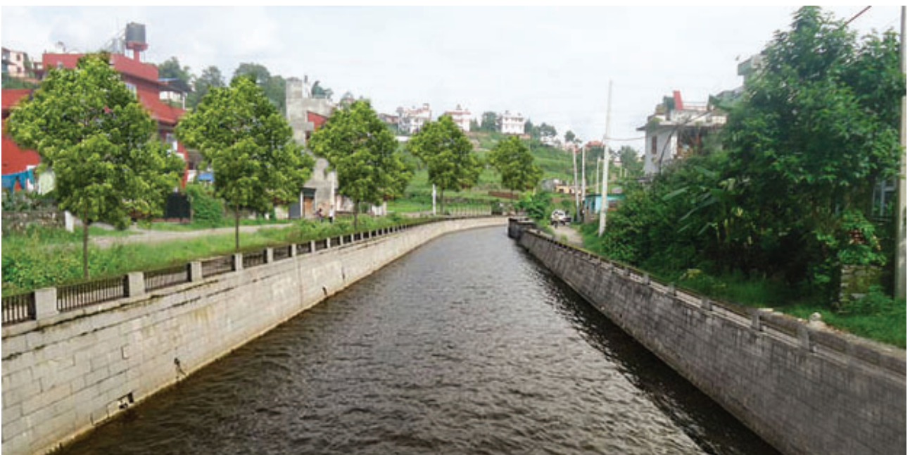
Figure 15: Dhobikhola at upper Kapan, After
