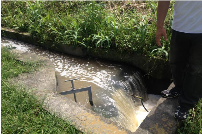
Figure 7: Outlet at the Gusheshwori WWTP before it connects to a sewer pipe that goes all the way till Tilganga.
